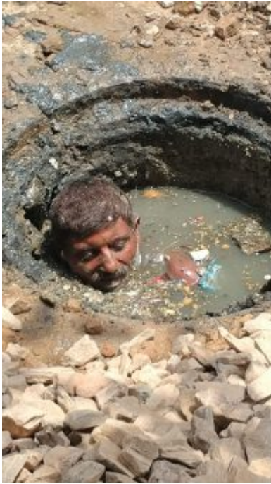
A sanitation worker is working inside a manhole to open sewer lines
